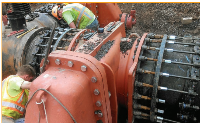
36" RW gate valve with EBAA split tandem megalugs
