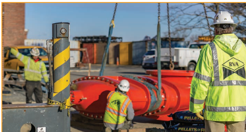
Bill Richardson, Jr. inspecting delivery of a 60" RW gate valve. (5) more 60", (2) 84" and (1) 132" gate valves to be commissioned at the MCUA Sayreville PS with NE Remsco.
