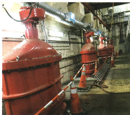
60" Resilient Seated Gate Valve. Made in the USA. Installed in Sayreville NJ
